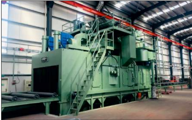
18 Turbine Shot Blasting Center
